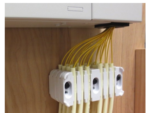
Microduct Manifold (cover removed)
